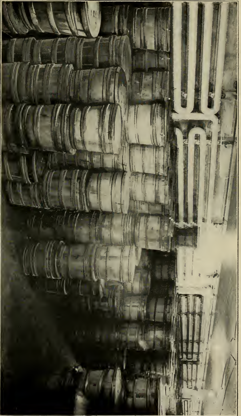
A MODERN "BUTTER BASEMENT", SHOWING REFRIGERATING PIPES THROUGH WHICH COLD AIR IS CONSTANTLY CIRCULATED
